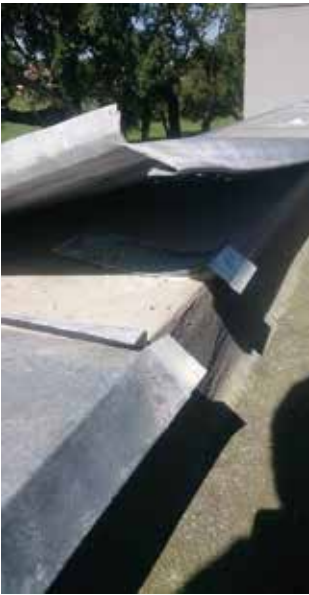
Corrosion of a zinc wall capping fixed directly over a cementitious material – easily and economically avoided by the use of a structural underlay (mat + breather) installed under the zinc
