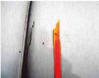
Wood chips and splinters absorb moisture, and can stay humid for enough time to mark the bright zinc surface. Care should also be taken with elZinc Alkimi®, Rainbow and Advance.
