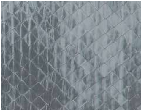
Staining caused by cleaning of adjacent brickwork by baking soda. These stains are difficult or impossible to remove without damaging the pre-weathered surface of Alkimi products, due to the chemical bonding of the contaminant to the surface. Depending on the aggressiveness of the cleaning products, also Rainbow and Advance finishes can be affected
