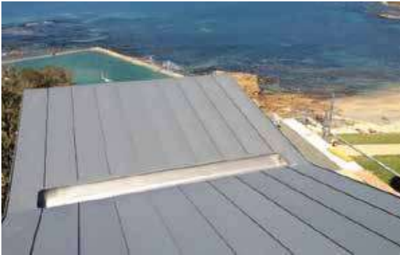
Frequently rain-washed areas do not allow salt deposits to build – elZinc Slate at Fairlight, Sydney
