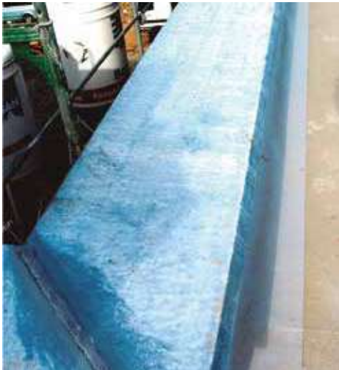
Staining caused by cement and plaster dust is costly to remove if it has stained the surface after light rain, fog or dew.
