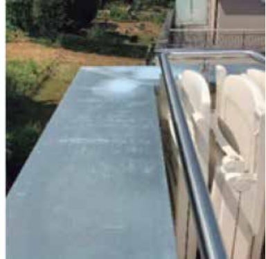
A more severe case due to ponding. Cases like this should be removed as soon as possible after they are detected.
