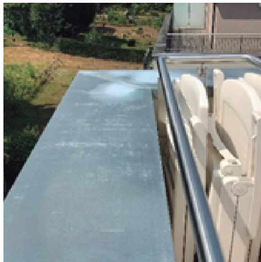
A more severe case due to ponding. Cases like this should be removed as soon as possible after they are detected.
