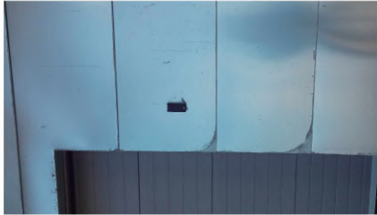
Partial removal of protective film causing differential weathering on natural zinc. These differences will weather-out over time
